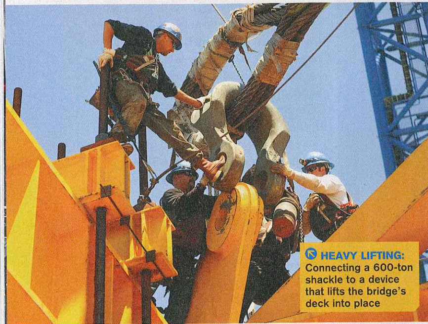
STRONG BASE: Installing the final pieces needed to build the bridge's foundation
