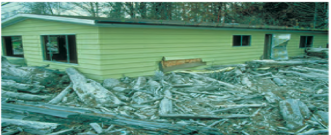
After the eruption of Mt. St. Helens, this home was damaged by a volcanic mudflow along the South Fork Toutle River in Washington state.
